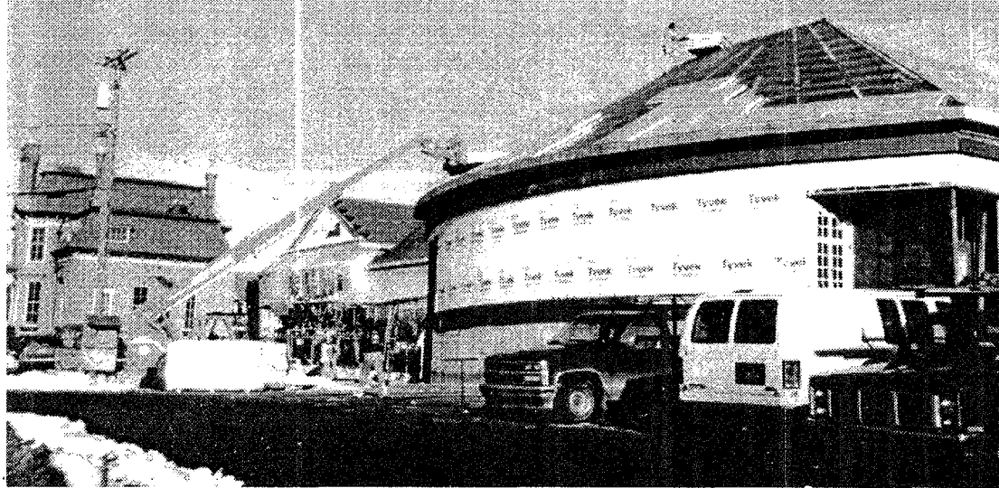
Tickets for safety violations issued to the contractor and subcontractors at the Plymouth Dunning-Hough Library construction site (above) have not slowed progress. The roof may be complete as soon as next week. (Crier photo by R. Alwood, Jr.).
